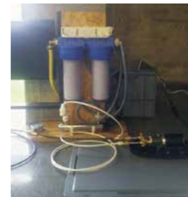
Fig 2: Pump + Filters A fog machine being used as pump
